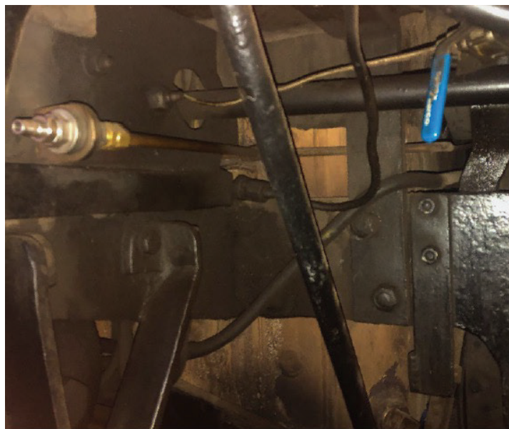
Shed air connection and steam separator drain valve (blue handle) under drivers-side tank.
