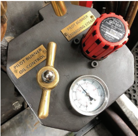
Pilot burner controls.
