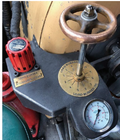
Load burner controls.
