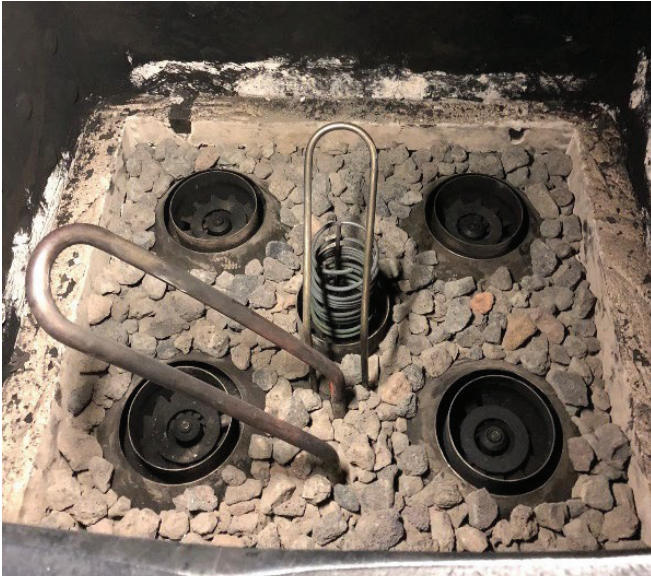
View of the burners through the firedoor.
